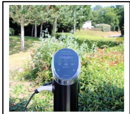
Public twin EV charger
