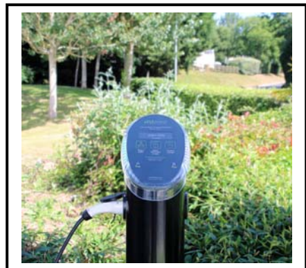
Public twin EV charger
